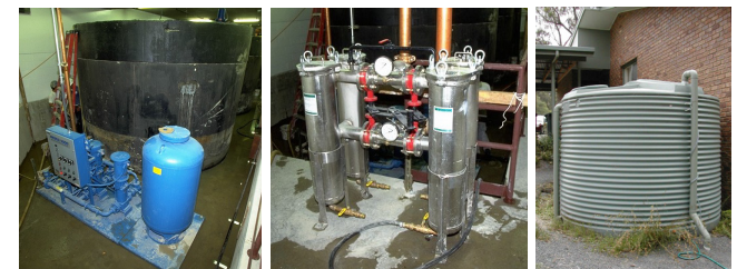
Figure 5: Examples of system components: pump, filter and tank.
